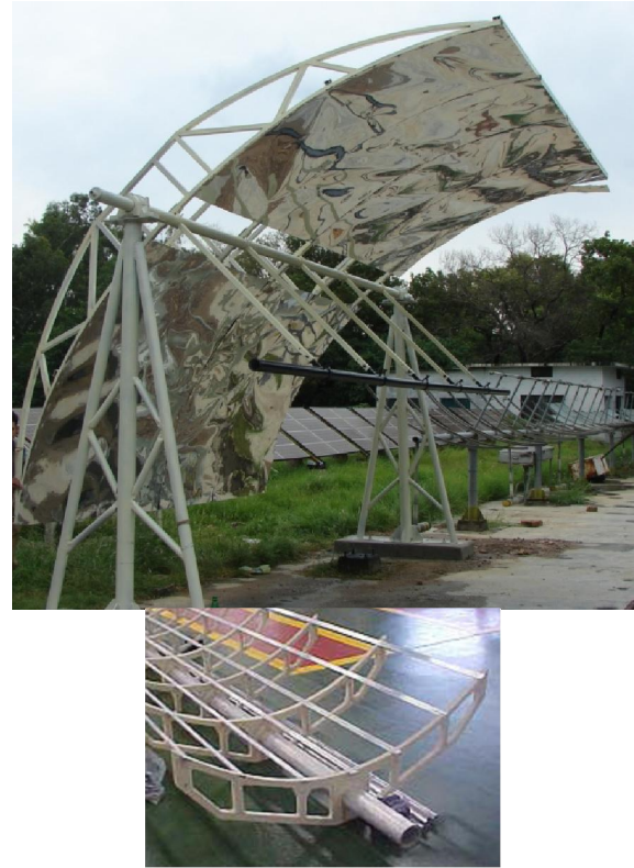
Fig.6 Structure of parabolic trough collector showing four steel ribs and Pylon
