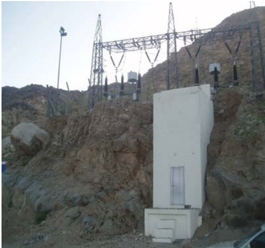
Fig 8: The landslide hazard at the installed electricity station of Al Aziziyah area, Makkah.
