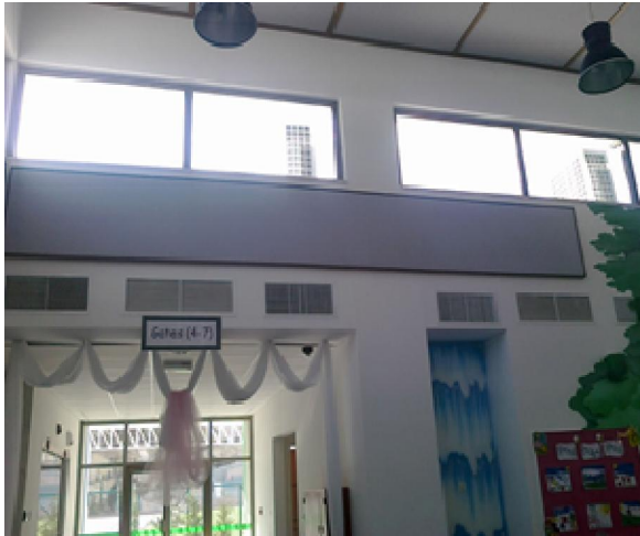
Figure 16. Sound proof panels on the walls
