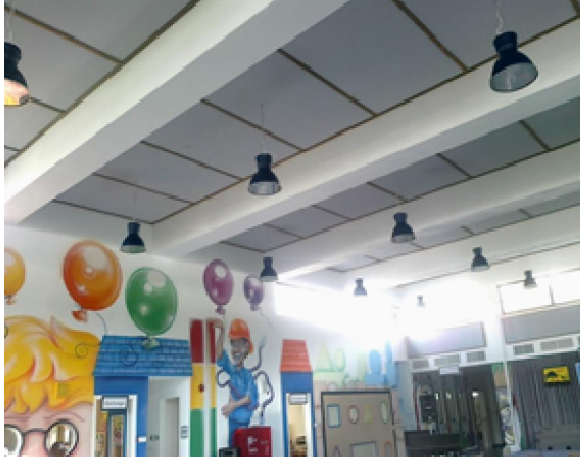
Figure 15. Wall decorations are kept the same after implementation of ceiling and wall sound proof treatment
