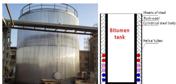
Figure 1. A Bitumen tank existed at INSUMAT Company, Tamouh – Giza, Egypt.
