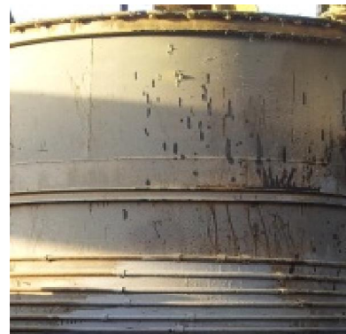
Figure 5. A snapshot of the worn Bitumen tank, before renovation.
